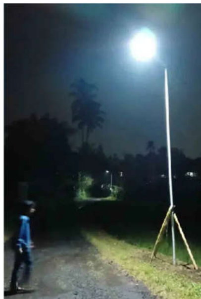
Fig. 3. Village street lighting with solar panels at night
