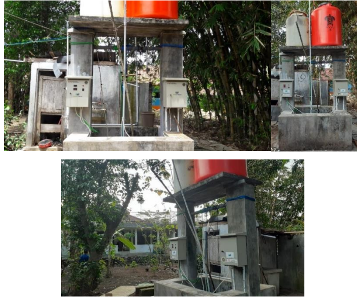
Fig. 9. Result of solar water pump
